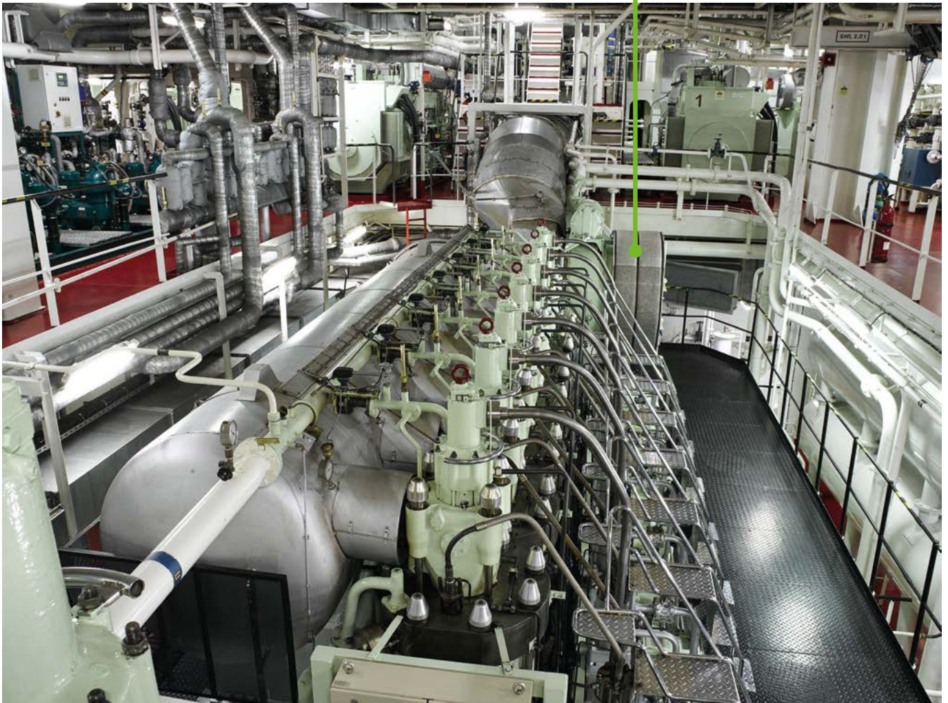
Air intake ship engine
